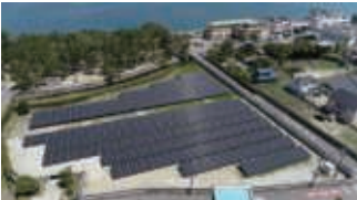
Solar power generating facilities (Tsuda, Sanuki City, Kagawa Prefecture) utilized by the Bank
